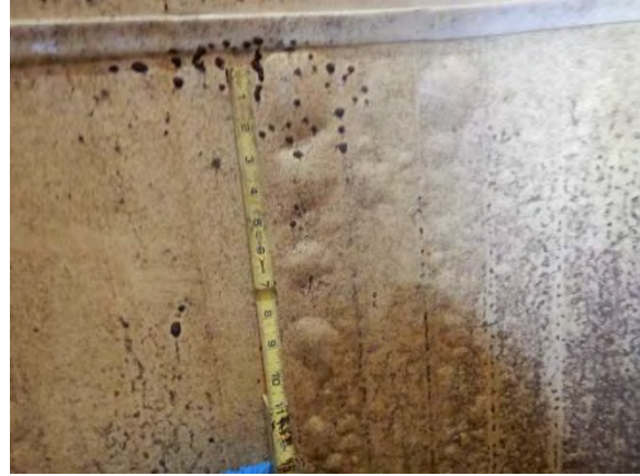
Photo 3-8. Typical blisters in lining on MAS walls.
