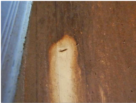
Photo 3-9. Cut in liner (only seen at 4D-4360 and 4D-0470).
