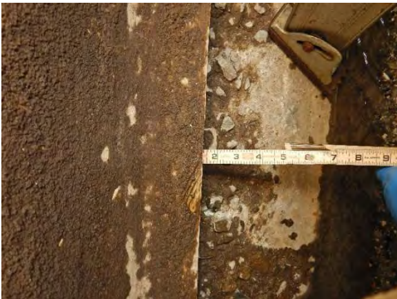
Photo 3-3. Typical lining termination undermined and unembedded.
