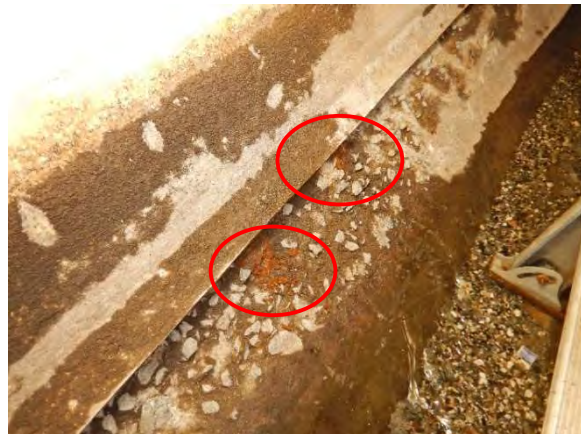
Photo 3-4. Reinforcement corrosion staining (only seen at 4D-0470)
