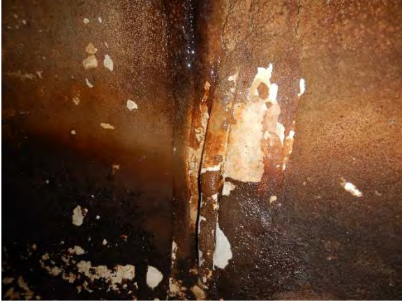
Photo 3-7. Typical failed weld strip.
