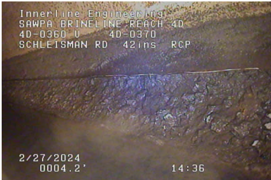
Figure 5: Exposed Aggregate and Liner Termination Uplift Between MAS 4D-0360 and 4D-0370
