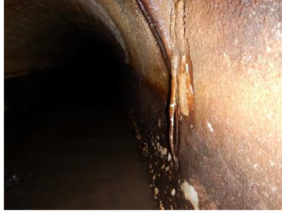
Photo 3-2. Failed weld strip (seen at 4D-0060 and 4D-0118).
