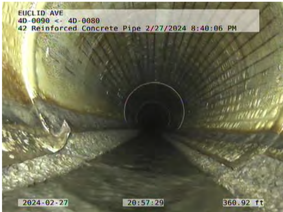
Figure 3: Rotated T-Lock Liner and Liner Detachment at Pipe Joint Between MAS 4D-0090 and 4D-0080
