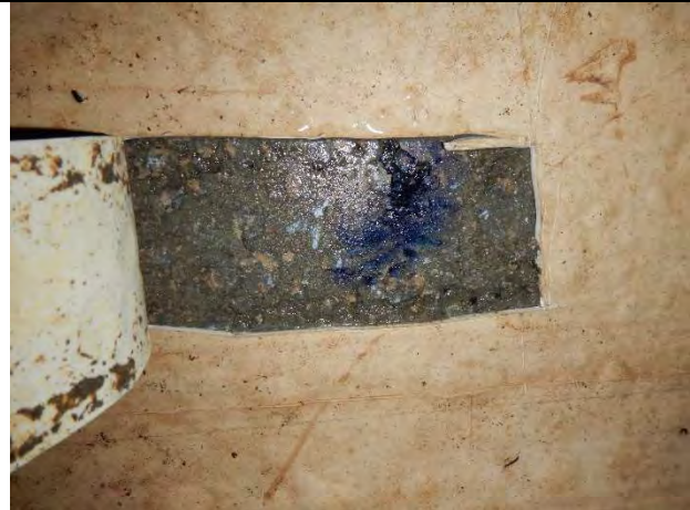
Effluent pipe liner cut at the crown (12:00)
