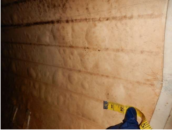
Photo 3-1. Typical lining blisters.
