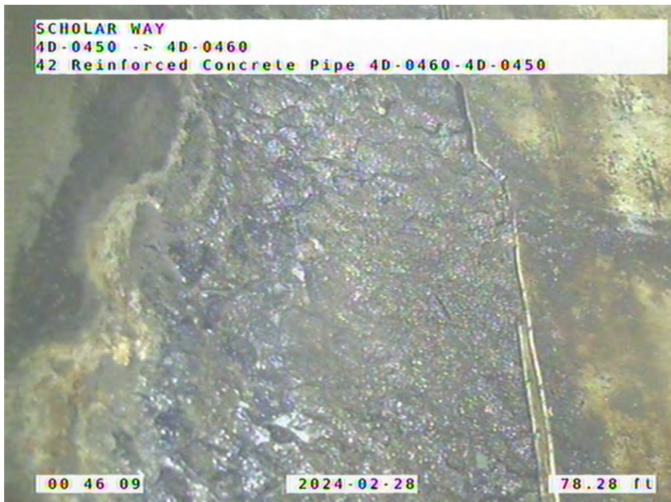
Figure 4: Minor Concrete Loss and Visible Aggregate Below Liner Termination Between MAS 4D-0450 and 4D-0460
