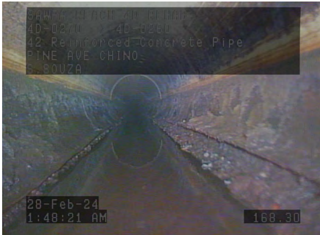
Figure 2: Liner Termination Uplift and Longitudinal Groove from Aggregate Loss Under Liner Between MAS 4D-0260 and 4D-0270
