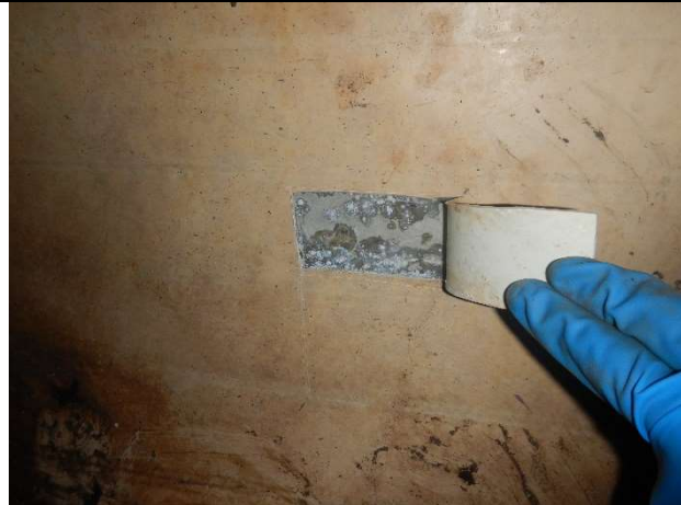
Influent pipe liner cut below the spring line (4:30)
