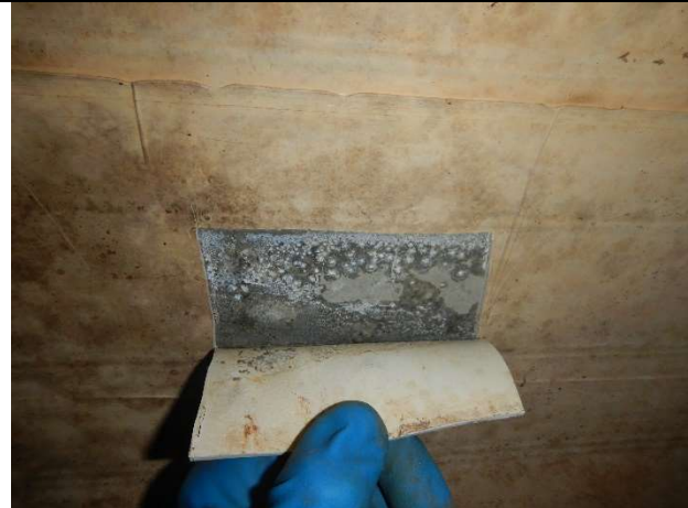
Effluent pipe liner cut at the crown (12:00)
