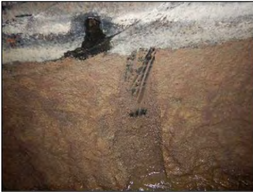
Figure 5: Typical Sediment Buildup
