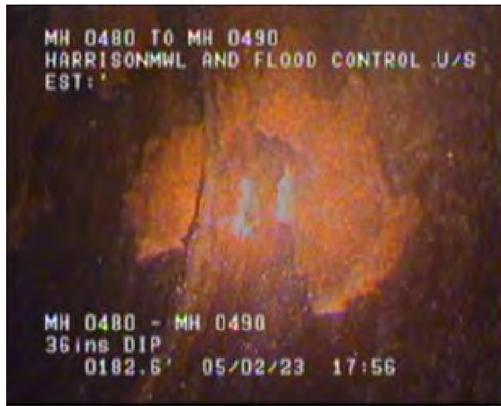
Missing Liner and Damaged Metallic Pipe Wall
