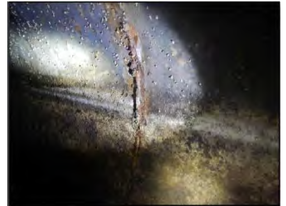
Coating Failure at Joint
