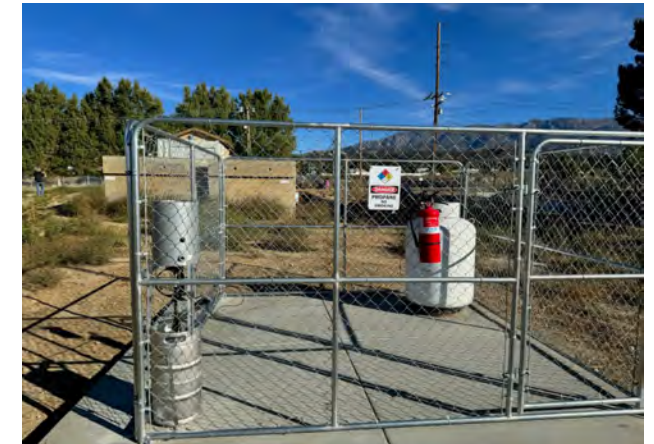
CNG unit with propane tank at site NE10
