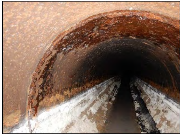
Figure 18: Moderate Corrosion (Looking Upstream)
