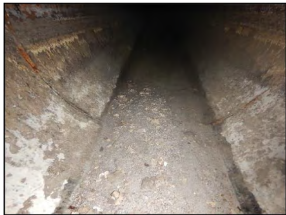
Figure 16: Sediment in Invert
