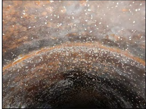
Figure 10: Corrosion at Crown
