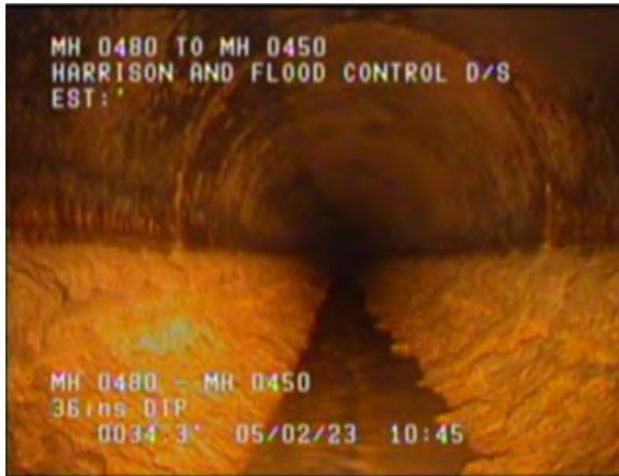
Figure 7: Deposits and Missing Liner
