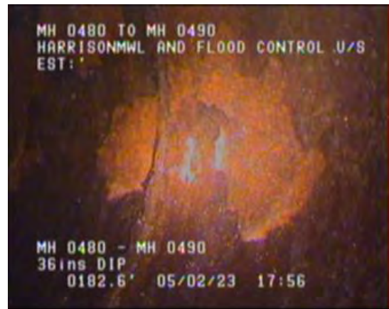
Figure 8: Missing Liner, Damaged Metallic Pipe Wall
