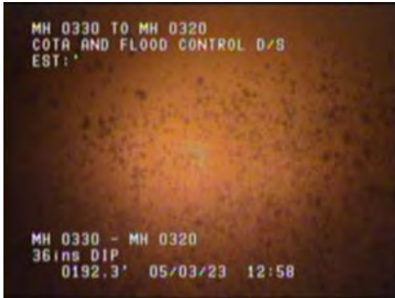
Figure 3: Early Corrosion Evidence at Pipe Crown
