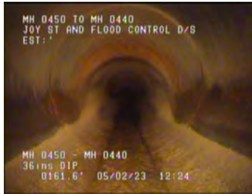
Corrosion Discoloration at Crown and Joint
