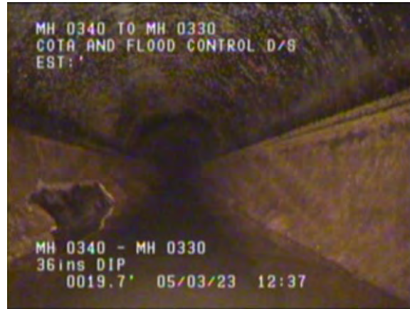
Figure 4: Missing Lining Material at 8 o'clock
