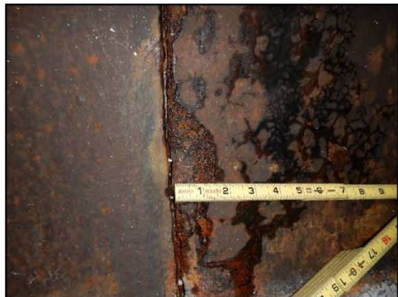
Figure 20: Coating Failure at Joint
