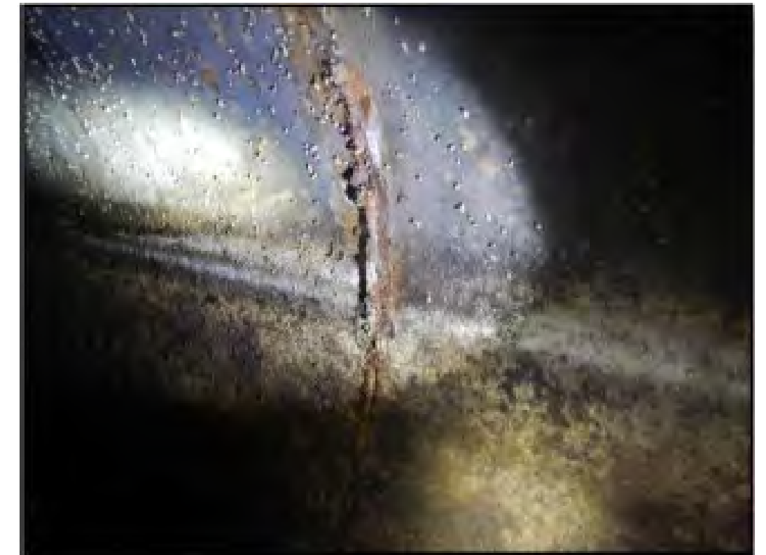
Coating Failure at Joint
