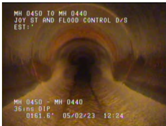
Figure 5: Corrosion Discoloration at Crown and Joint
