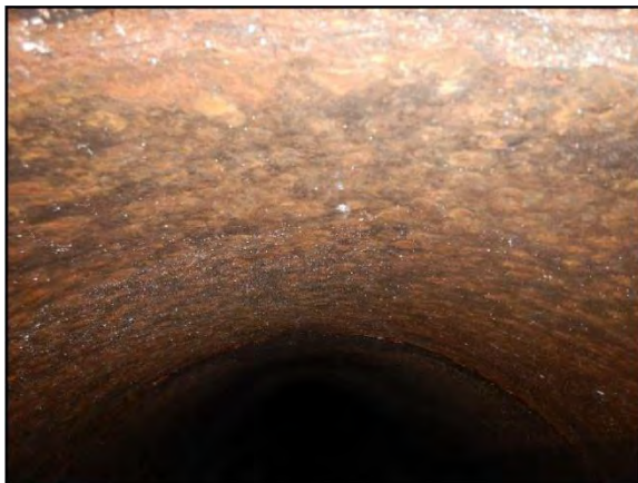
Figure 19: Moderate Corrosion at Crown
