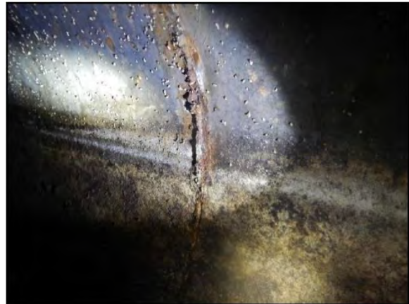
Figure 12: Coating Failure at Joint
