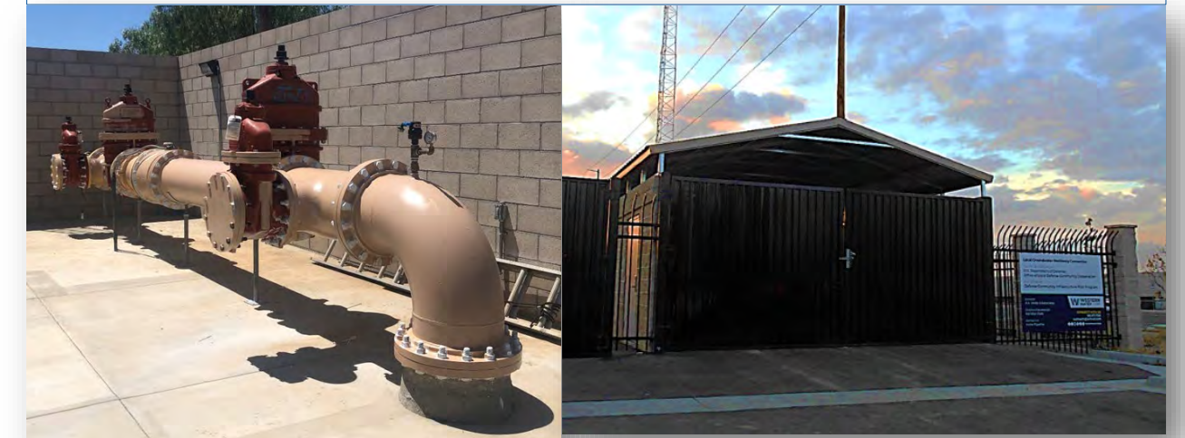
MARB Interconnection Facility
