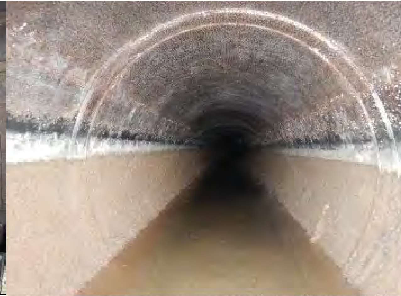
Up to 1/4" of sediment observed on pipe walls
