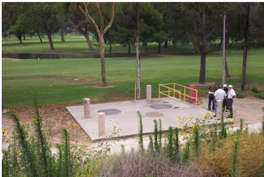
(4) Looking southwest. View of golf course access road and Green River metering vault.
