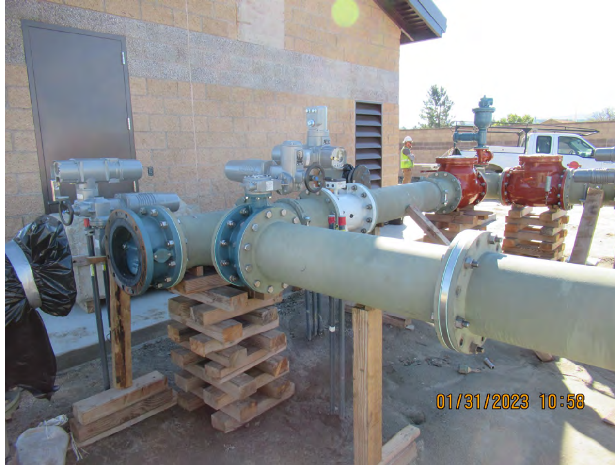
Well 201 Piping, January 2023
