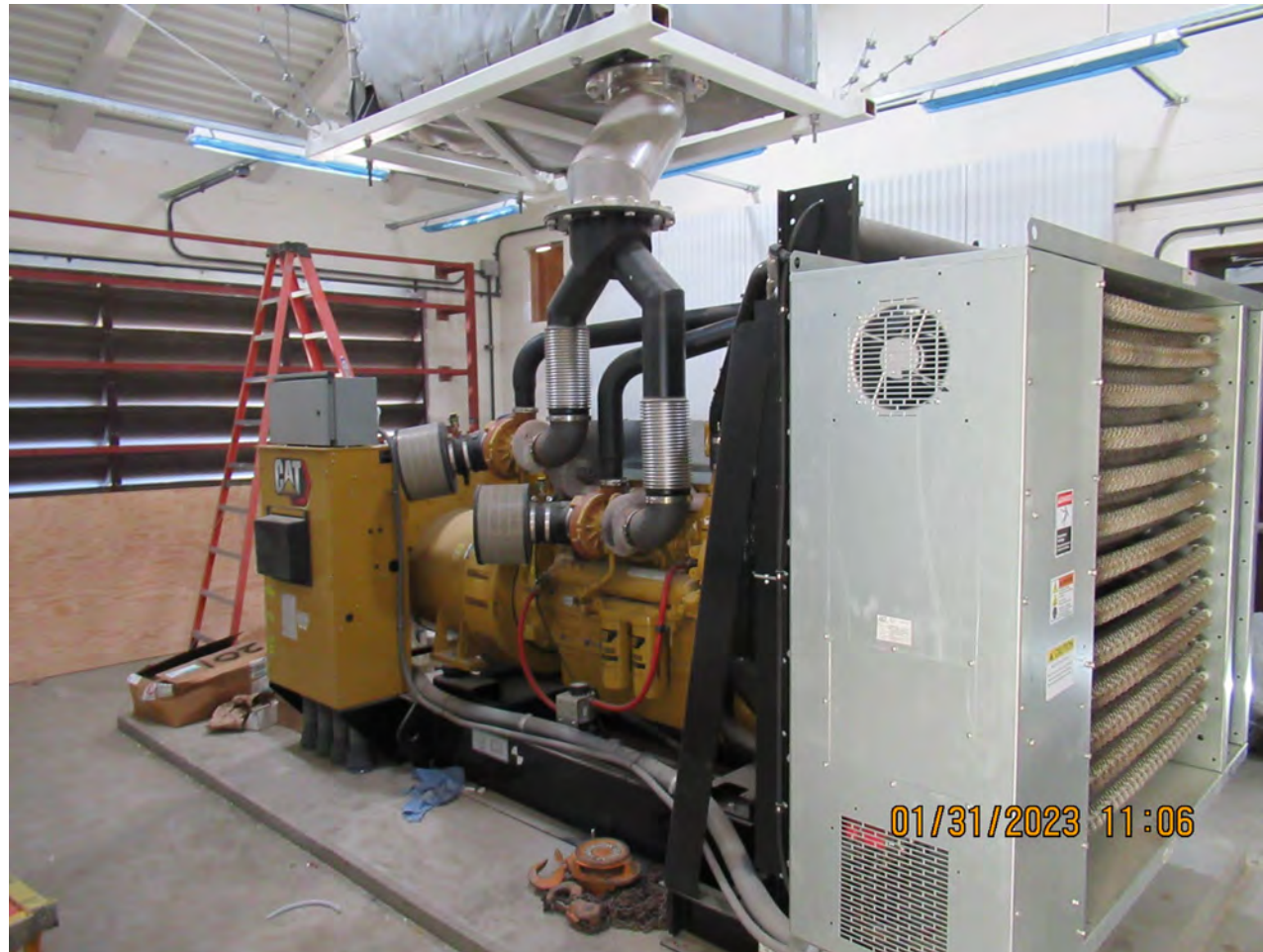
Well 201 Generator, January 2023
