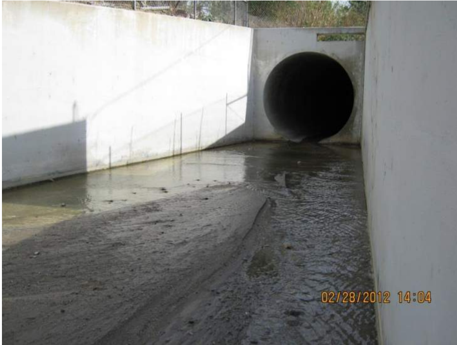
Storm drain outlet.
