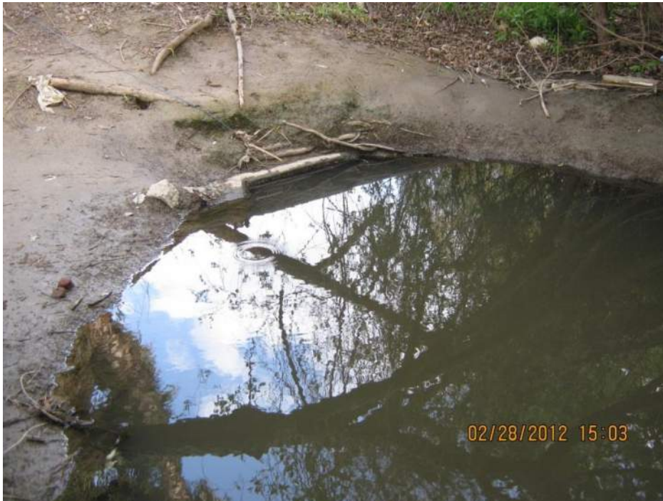
Ponded water from outfall, visible structure assumed to be ceiling of outfall.
