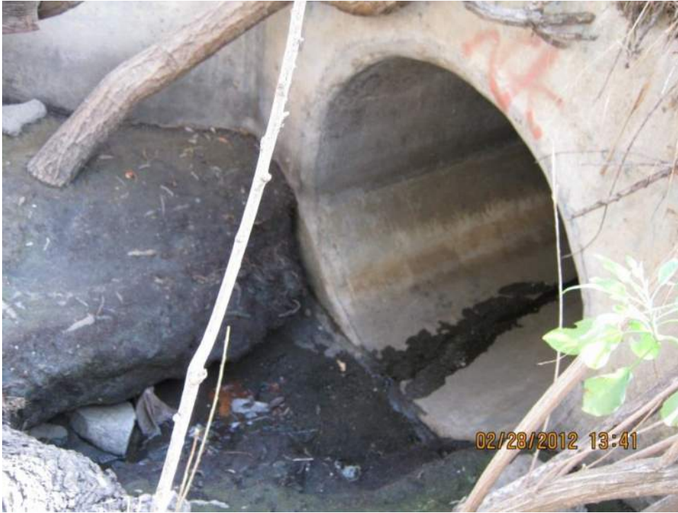
Outfall pipe with trickle flow.
