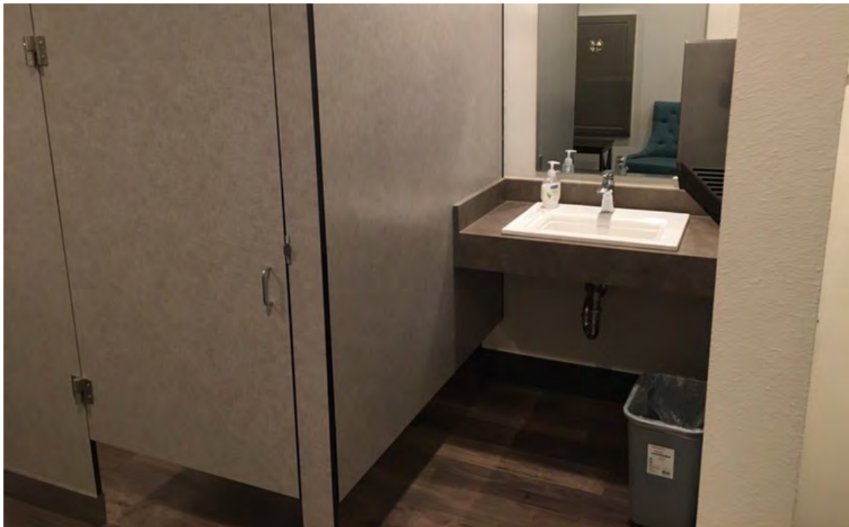
B2 PHOTO B2- Existing Lavatory at Women's Restroom (Lack of Pipe Wrapping) | First Floor
