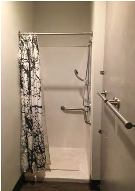
D2 PHOTO D2- Existing Non-Compliant Shower | First Floor
