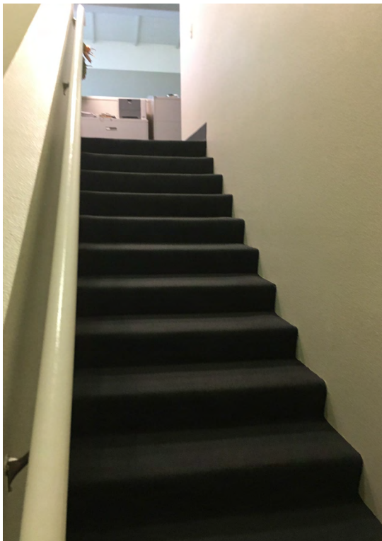
C3 PHOTO C3- Missing Handrail at Stair
