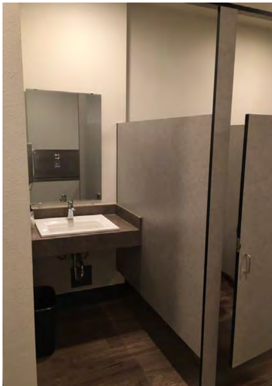
H2 PHOTO H2- Existing Lavatory at Men's Restroom (Lack of Pipe Wrapping) | First Floor
