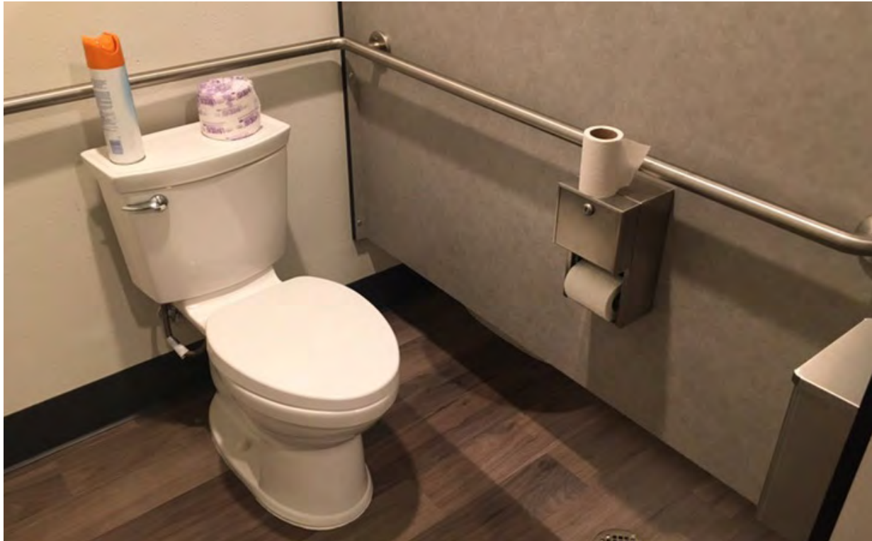
C2 PHOTO C2- Existing Accessible Stall with Continuous Grab Bars | First Floor
