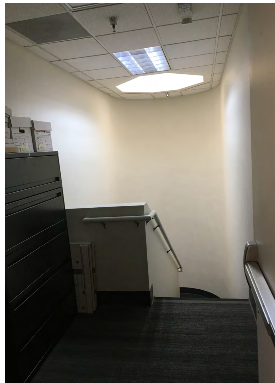
D3 PHOTO D4- Missing Handrail at Stair
