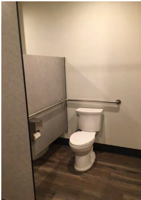
K2 PHOTO K2- Existing Accessible Stall with Continuous Grab Bars | First Floor
