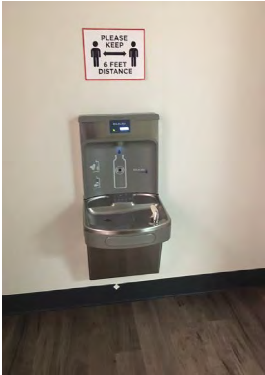
F2 PHOTO F2- Existing Drinking Fountain (Lacking Hi-Lo Fountain per ADA)
