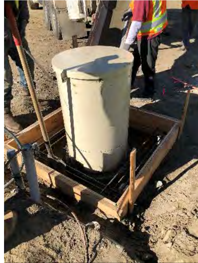
Monitoring Well MP-01
