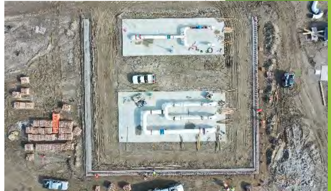
Mechanical Piping Pads
