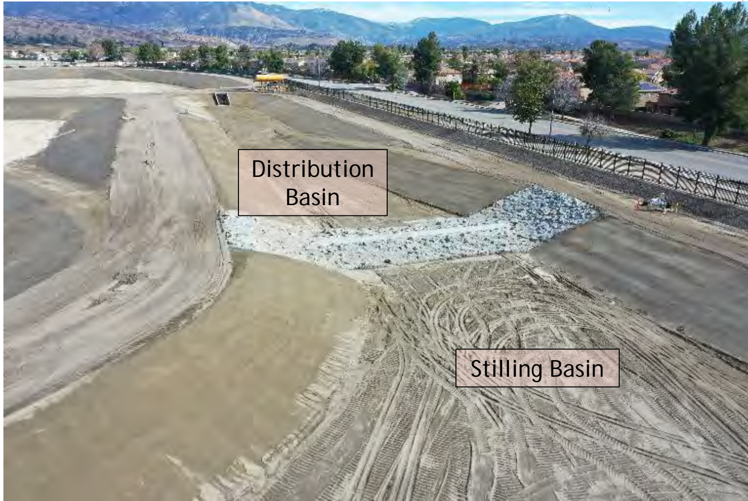
Weir between stilling basin and distribution basin
