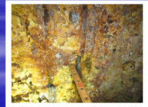
MAS Concrete Deterioration
