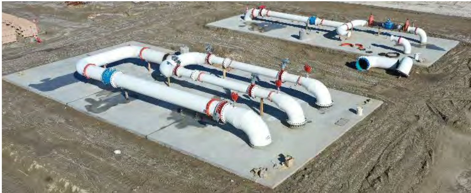
Raw Water Inlet Piping
