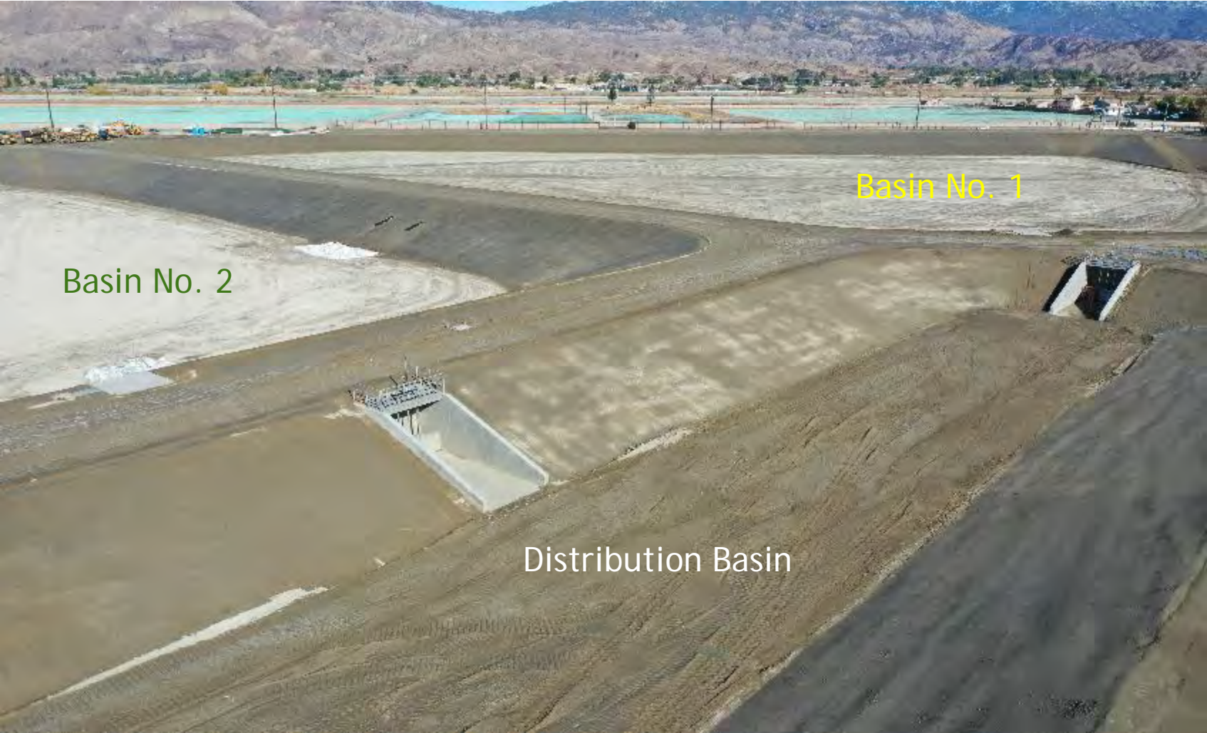
Distribution Basin and Outlet Control Facilities
