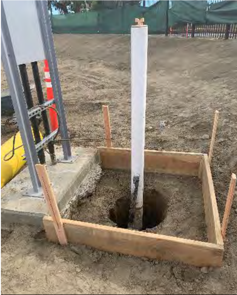
Shallow Monitoring Well
