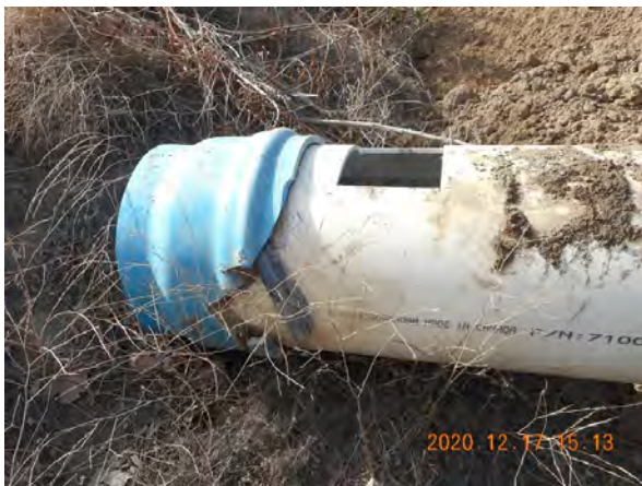
Figure 2. Damaged Pipe Bell.
