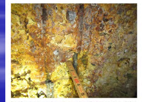
MAS Concrete Deterioration
