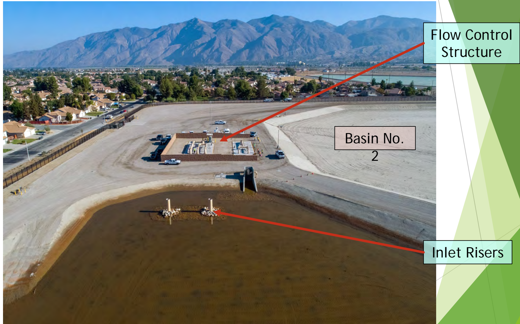
Aerial View of Mechanical Piping and Stilling Basin
