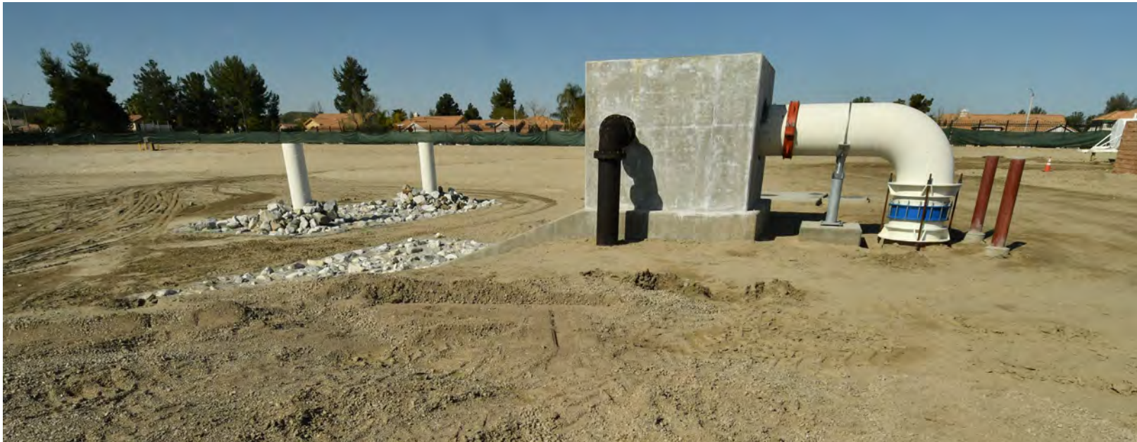
Water Outlet Pipes and Stilling Basin
