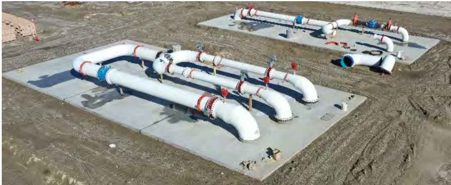
Raw Water Inlet Piping
