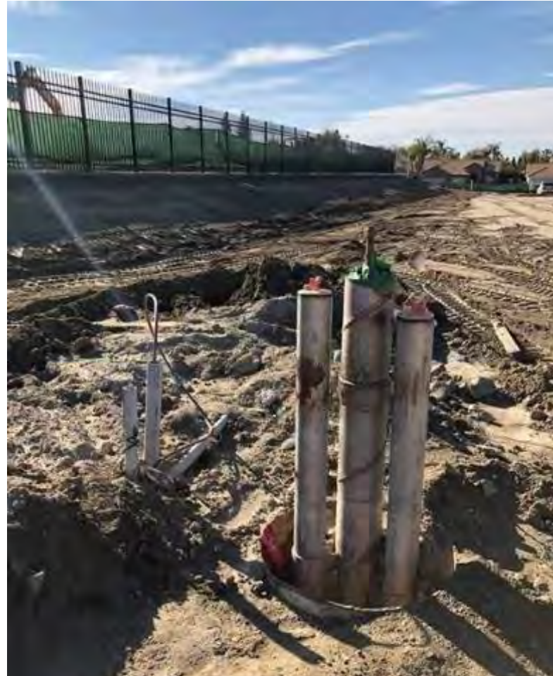
Monitoring Well MP-01
