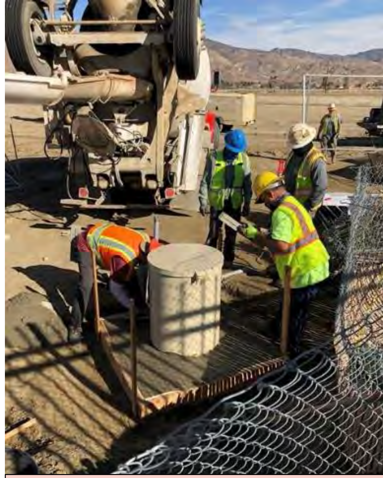
Monitoring Well MP-03
