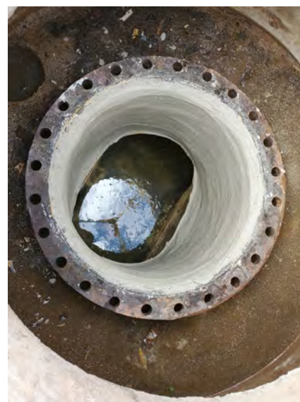
Figure 4 – Structure prepared with a layer of mortar prior to reapplying an epoxy-based liner.
