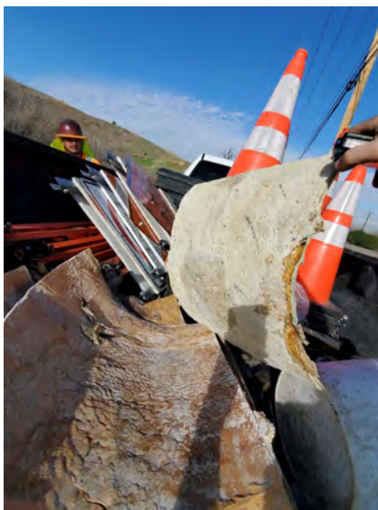
Figure 3 – Removed section of spray-on liner.
