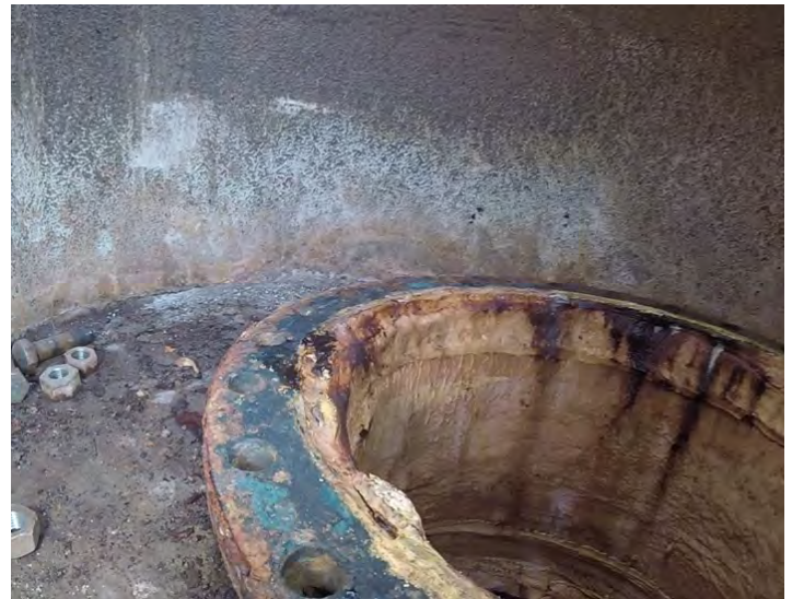
Figure 2 – Maintenance Access Structure. Note damage to existing spray-on liner.
