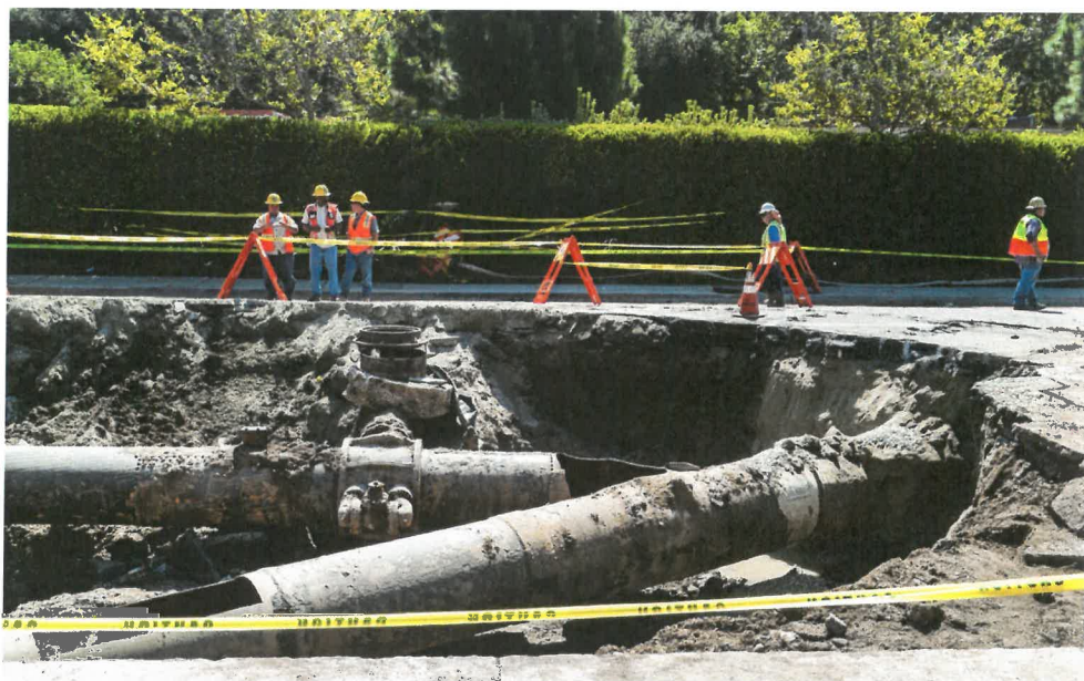
Los Angeles Department of Water and Power crews work to repair a water main that ruptured on Sunset Boulevard in July 2014. The pipe was 93 years old. (Damian Dovarganes, AP)
