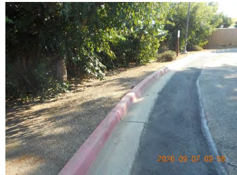
Figure 2. North side of the SAWPA Parking Lot. The WMWD SCADA conduit was installed adjacent to the existing curb and gutter.
