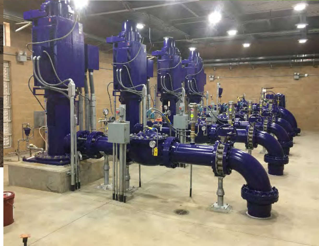
Sterling Pump Station Finalizing electrical and instrumentation to commence facility startup testing
