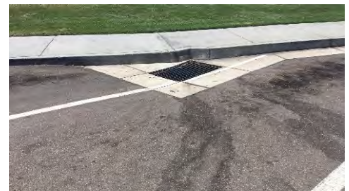
Dry Weather Inspection, Pollution Release Identified
