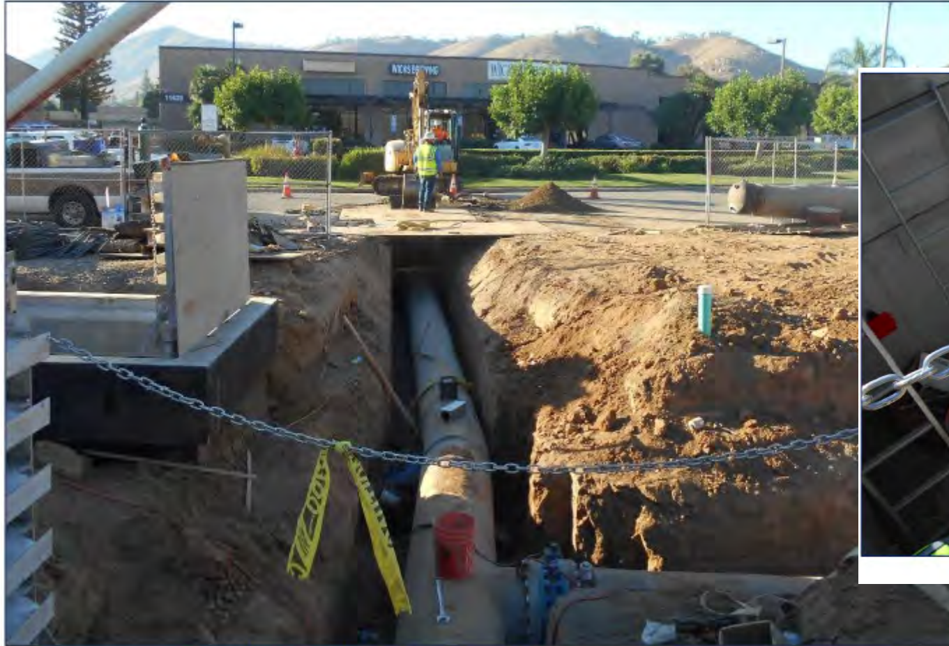
Installation of Pipe B into Sterling Avenue / Connection of Pipes B and C
