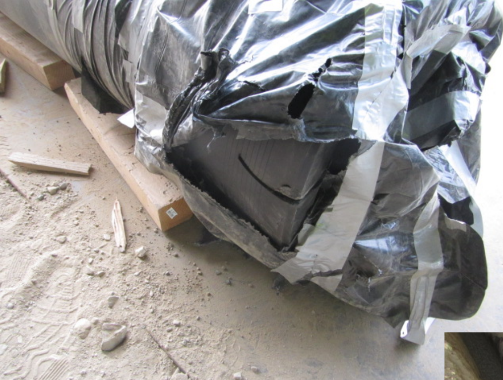
Damaged EF coupling
