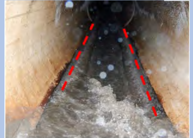
Photo 3-6. Steep slope for Manhole 4D-0150 influent pipe. Apparent typical water level indicated by red
