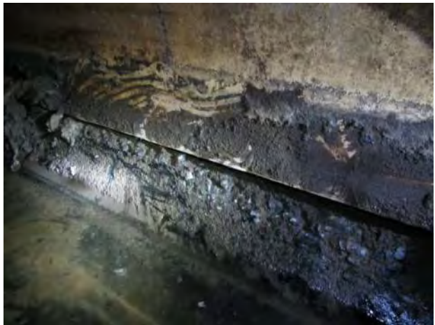
Photo 4-7. Typical undermined liner termination and exposed aggregate.
