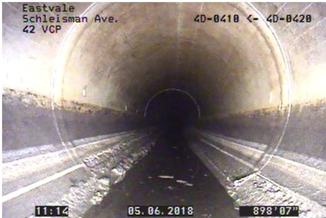
Figure 3: Rotated T-Lock Liner at Pipe Joint Between MAS 4D-0410 and 4D-0420
