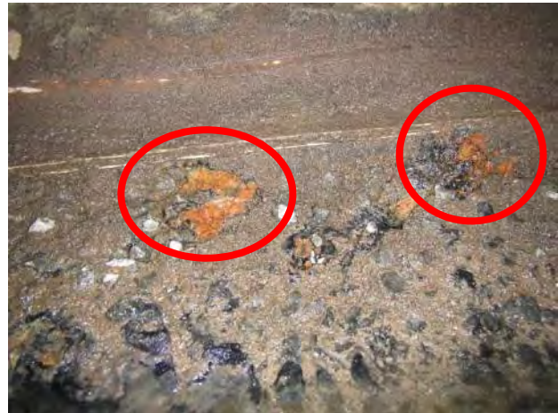
Photo 3-4. Exposed reinforcing steel only seen at Manhole 4D-0470 (circled in red).
