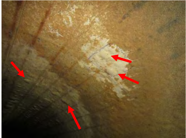
Photo 3-1. Typical lining blisters (indicated by red arrows).
