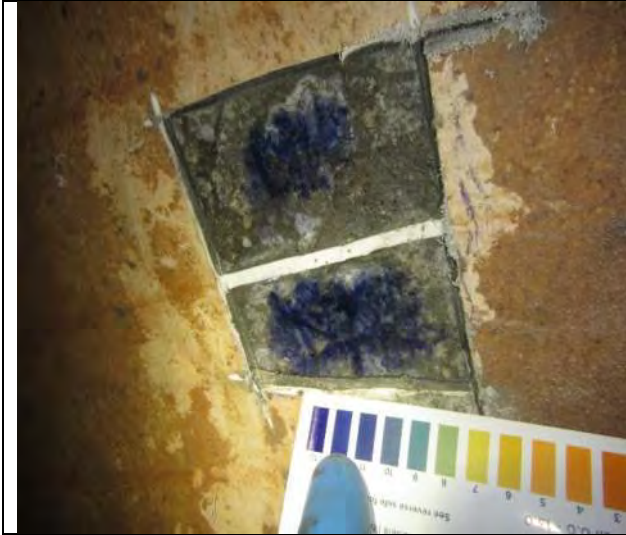
Influent pipe liner cut at crown (11:00)
