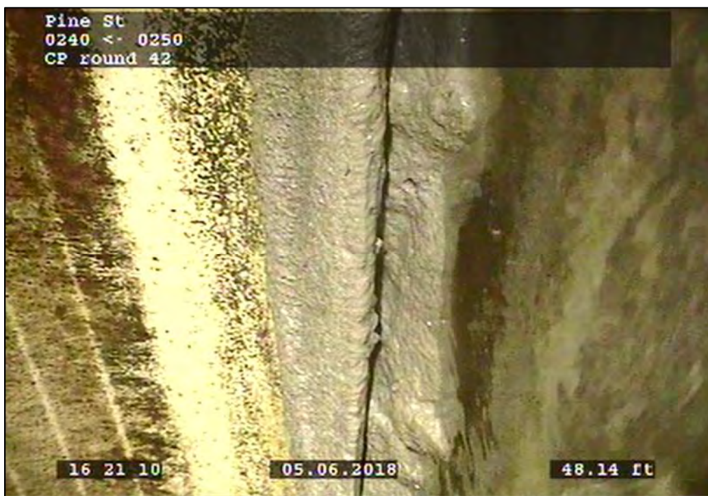
Figure 6: Liner Termination Uplift Along Pipe Segment Between MAS 4D-0240 and 4D-0250
