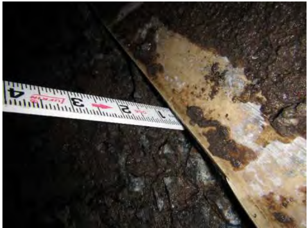
Photo 3-3. Typical undermined and unembedded liner termination. Typical exposed concrete aggregate.
