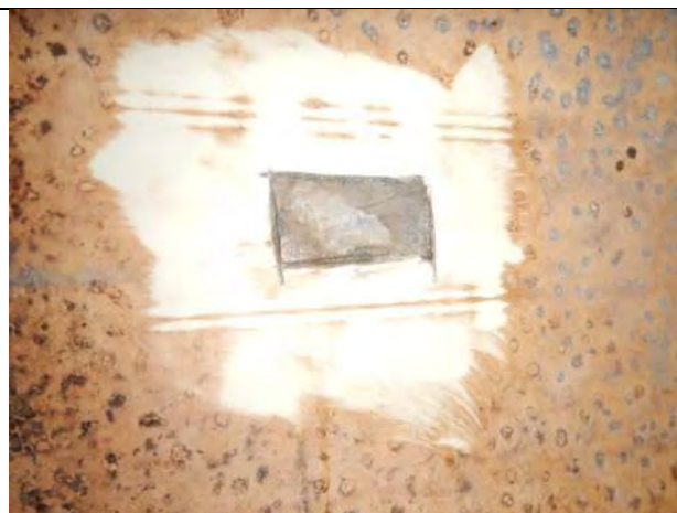
Effluent pipe liner cut at spring line (9:00)
