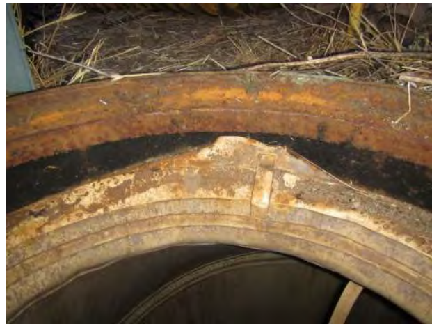
Photo 4-4. Typical loose liner termination.
