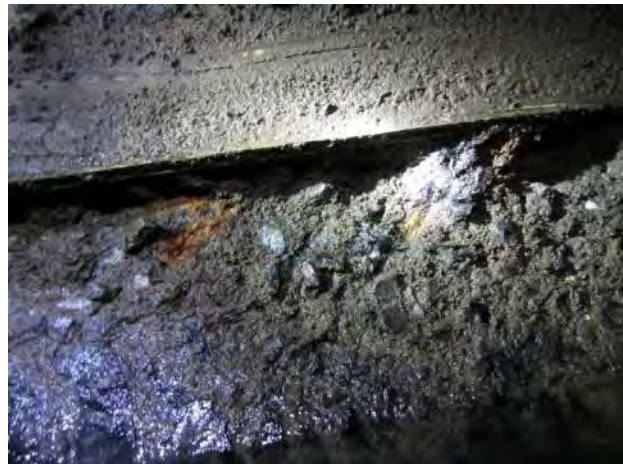
Photo 4-8. Exposed reinforcing steel only seen at MH 4D-0470.
