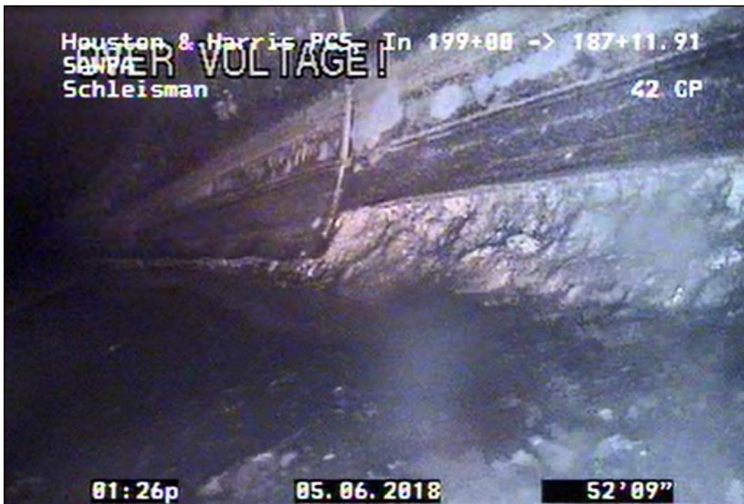
Figure 5: Minor Concrete Loss and Visible Aggregate Below Liner Termination and Rotated T-Lock Liner at Pipe Joint Between MAS 4D-0380 and 4D-0390
