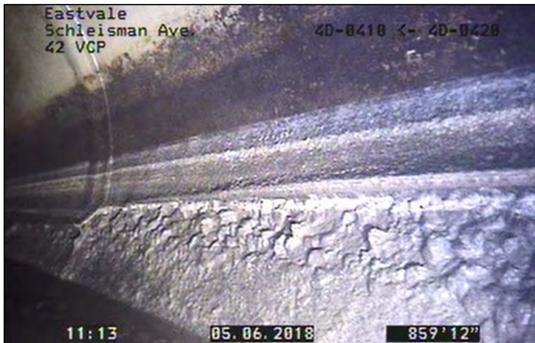
Figure 4: Minor Concrete Loss and Visible Aggregate Below Liner Termination and Rotated T-Lock Liner at Pipe Joint Between MAS 4D-0410 and 4D-0420
