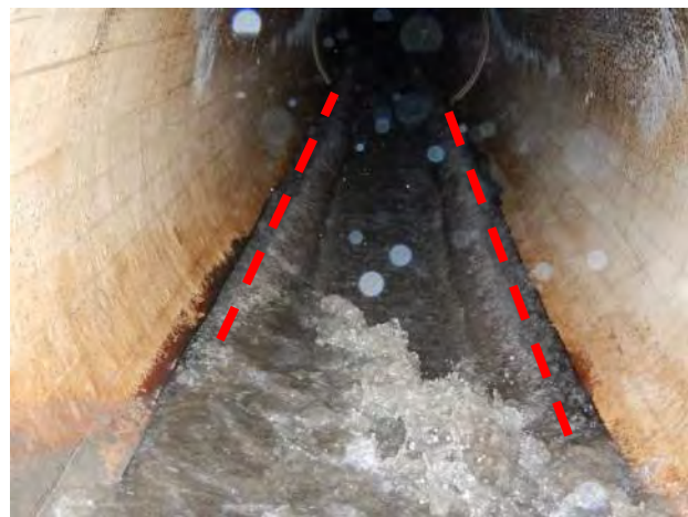
Photo 3-6. Steep slope for Manhole 4D-0150 influent pipe. Apparent typical water level indicated by red
