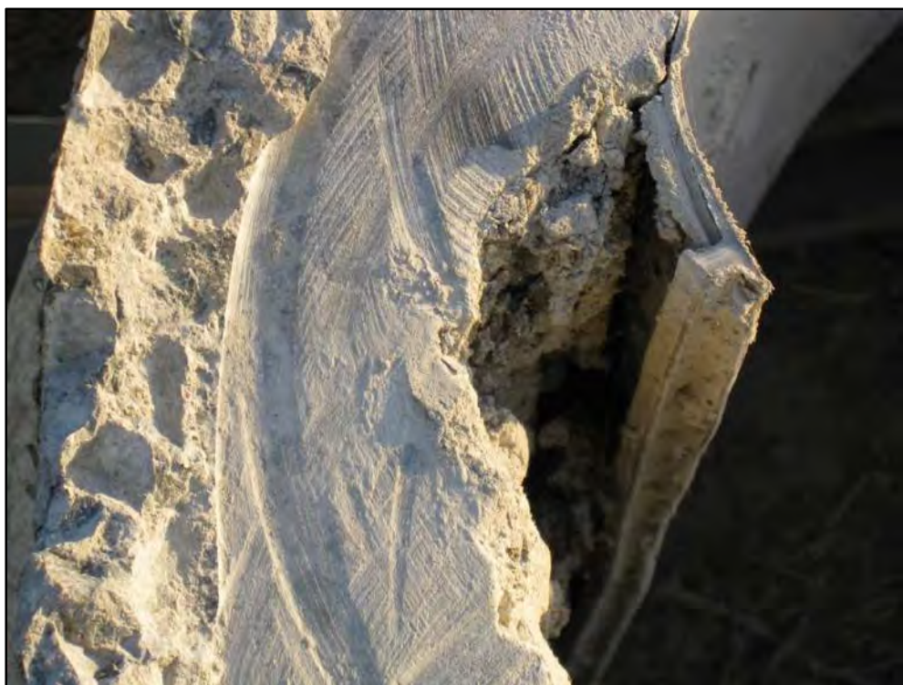
Figure 2: Concrete deterioration and uplifting of T-Lock liner in section of RCP removed in 2011. Photo Courtesy of SAWPA.
