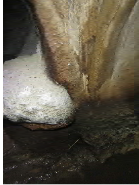
Photo 4-2. Typical slime layer and encrustation.
