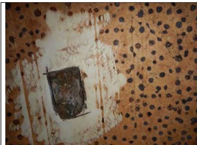
Effluent pipe liner cut at crown (12:00)
