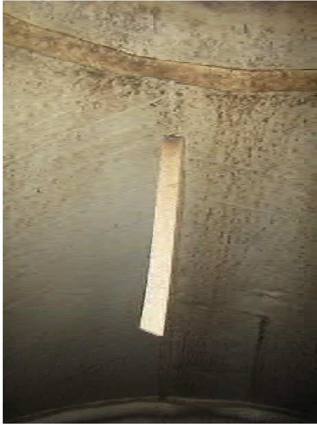
Photo 4-1. Typical failed liner weld strip.
