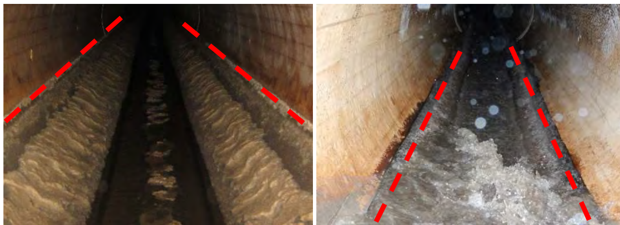
Figure 7: Typical Water Level (dashed red line) Indicated by Slime Layer (Left). Typical Water Level (dashed red line) in Steep Slope Between MAS 4D-0160 and 4D-0150 (Right).
