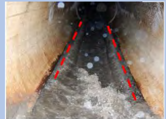
Photo 3-6. Steep slope for Manhole 4D-0150 influent pipe. Apparent typical water level indicated by red
