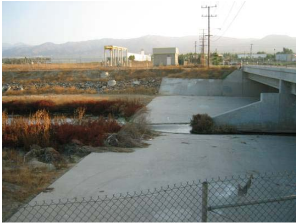
Figure 59 Temescal Creek transitions from concrete lined to natural below Lincoln Avenue Bridge
