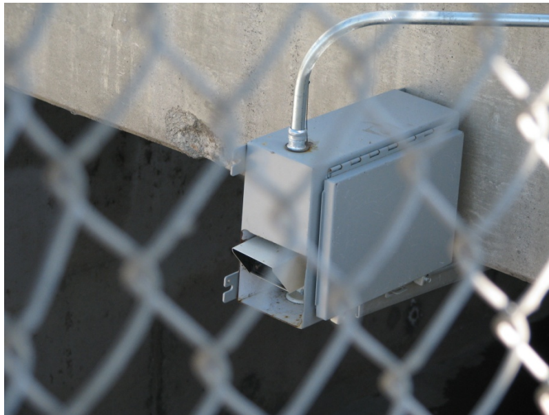
Figure 3 Photo of the Recreational Use Survey Camera Installation for Demens Channel
