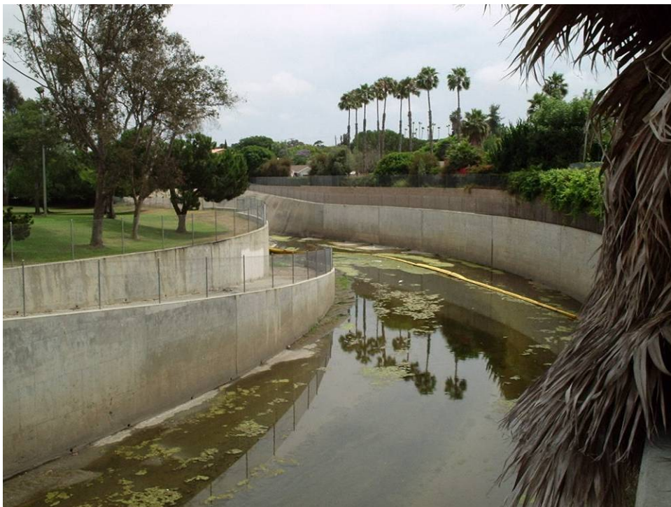
Figure 2b Photo of the Santa Ana Delhi Channel at the Mesa Avenue Recreational Use Survey Location
