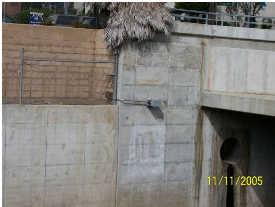
Figure 3b Photo of the Santa Ana Delhi Channel at the Mesa Avenue Recreational Use Survey Camera Installation
