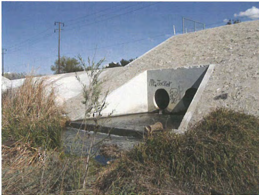
Evans Lake Channel, view of culvert and drop structure just below confluence of channel and SAR.
