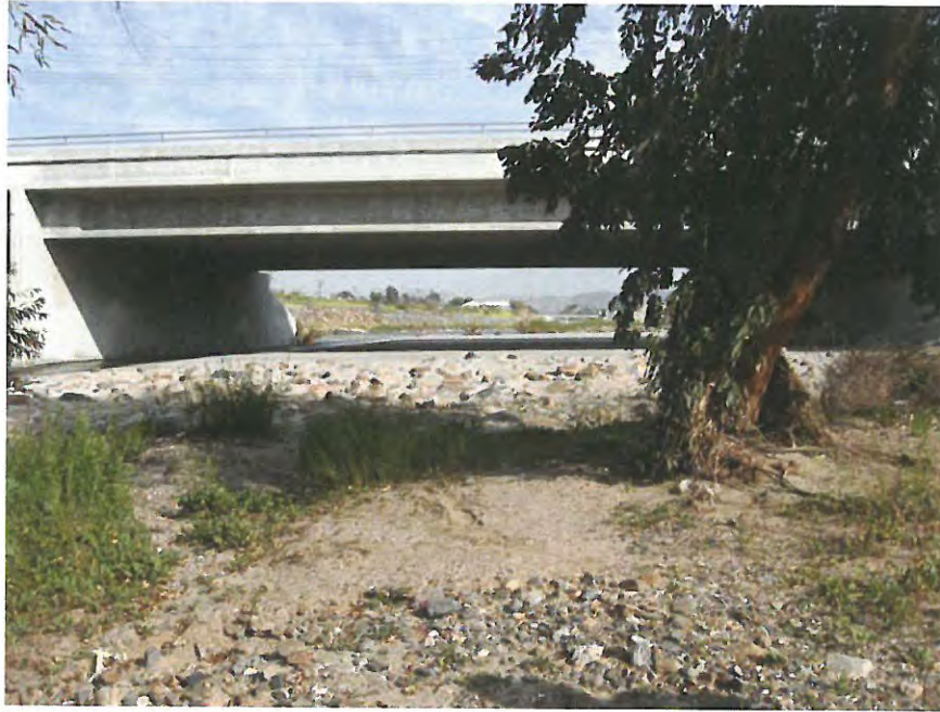
Temescal Creek, concrete lined flood control facility upstream of Lincoln Avenue crossing.
