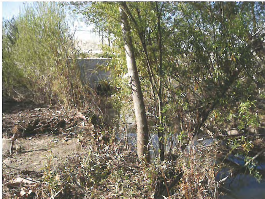
Evans Lake Channel, surface flows conveyed through culvert to SAR.
