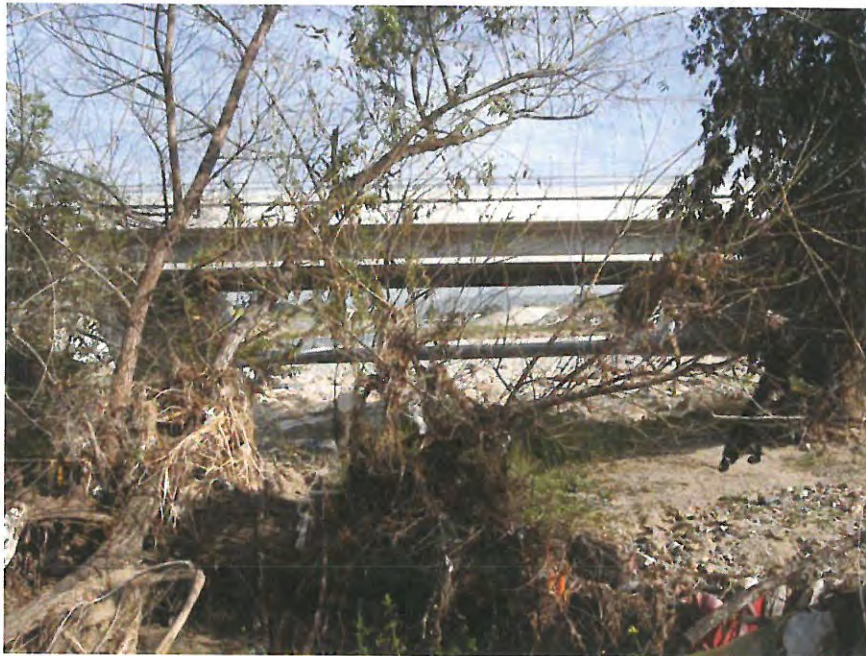
Temescal Creek, immediately downstream of Lincoln Avenue crossing. Heavy debris in creek.
