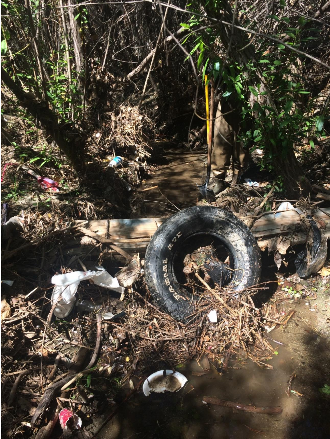
Figure 5: Trash debris buildup after a storm event.
