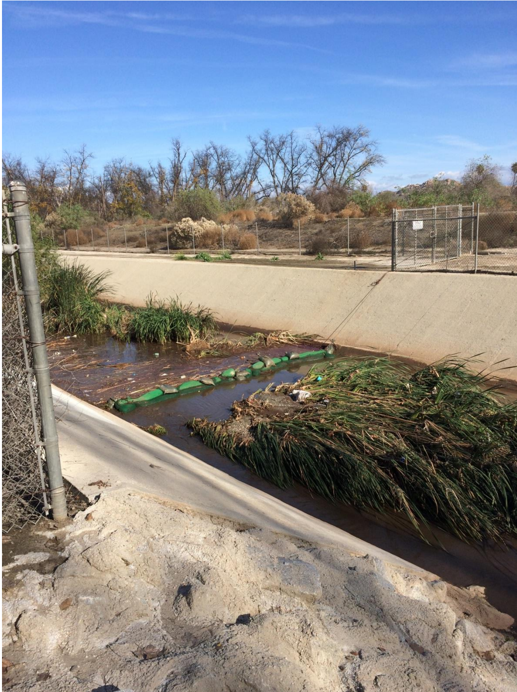
Figure 4: Riverside County Flood Control check dam set in place to prevent sediment and trash from entering creek while removing vegetation from concrete-lined channel.
